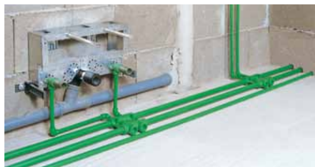
Floor distribution with distribution blocks
